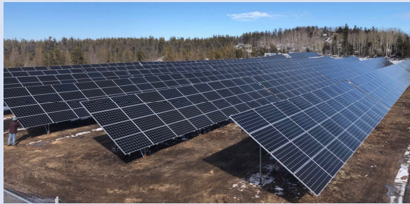
Figure 7.3: Ft. Chipewyan Solar Farm
